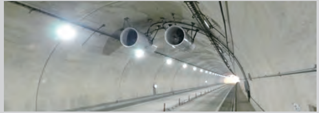
各種トンネル設備(受変電・照明・防災・換気・通信設備等)の設計 Tunnel facilities (Power receiving and transforming facilities, lightning, disaster prevention, ventilation, telecommunication systems)
