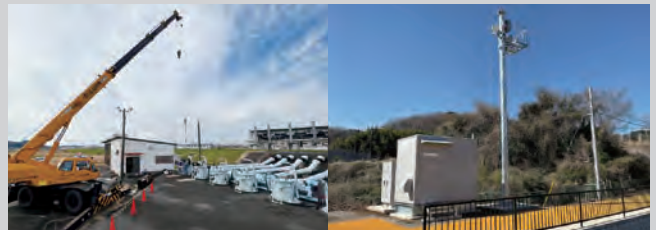
河川用機械設備(排水ポンプ、ゲート)の設計、治水関連設備(遊水地遠隔監視設備)の設計 A design of mechanical equipment for flood control, (pump, gate, telecontrol and telemeter, etc.)
